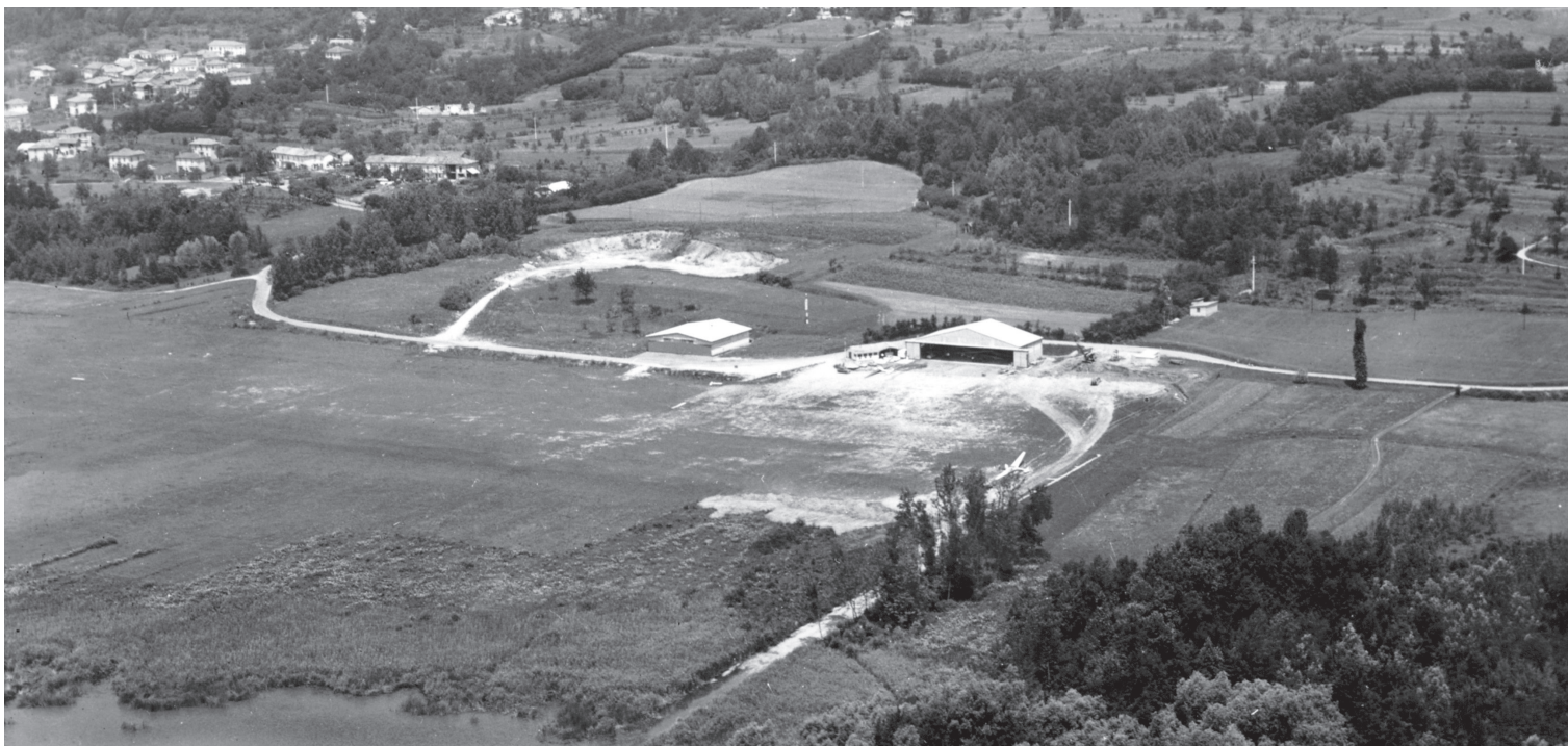
I lavori a Calcinate con i primi hangar • The various phases of the works in Calcinate with the first hangars
